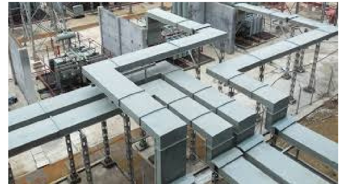
Bus-Bar Trunking System (BBT)
