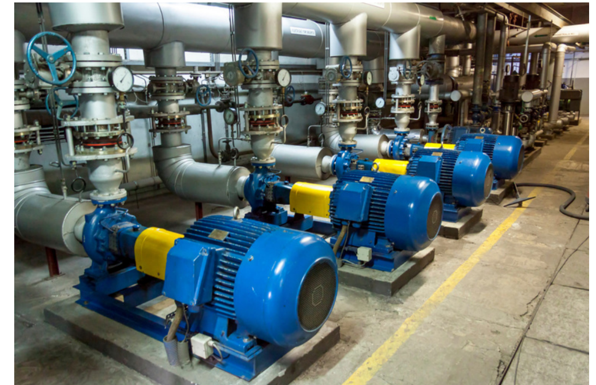
Pumps & Pumping System:
